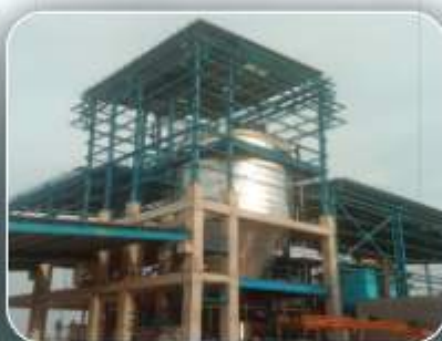
ATOMIZER PLANT CAPACITY 1 KL PER HOUR
