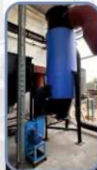
AIR PRE HEATER
