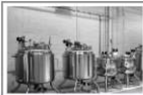
TANKS AND VESSELS
